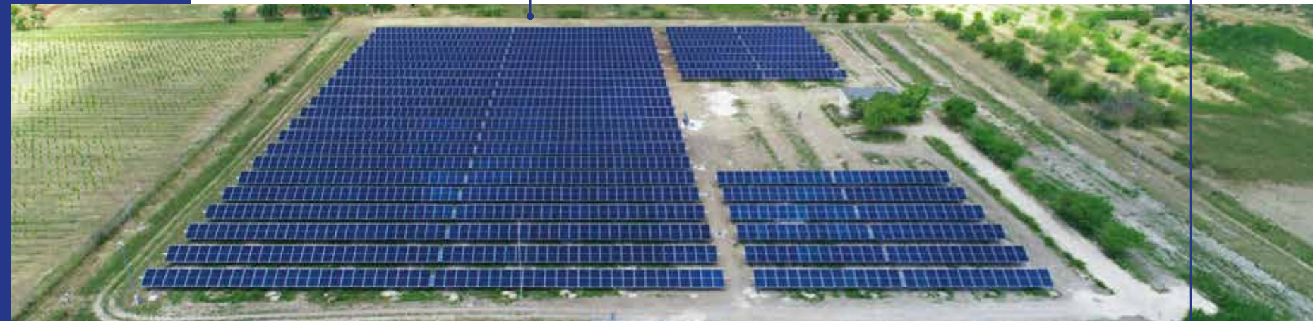
Photovoltaic Park of Ruvo di Puglia in the Polvino district
